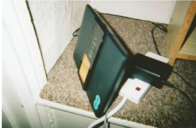
Fig.1 Accessibility - Wireless Network Router
